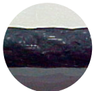
Lubricating covering broken wires making inspection impossible
